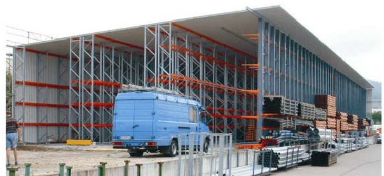
Fig. 3: Combined racking shed consisting of ELVEDI pallet and cantilever racking, building under construction. The racking is designed to carry walls and roofing
